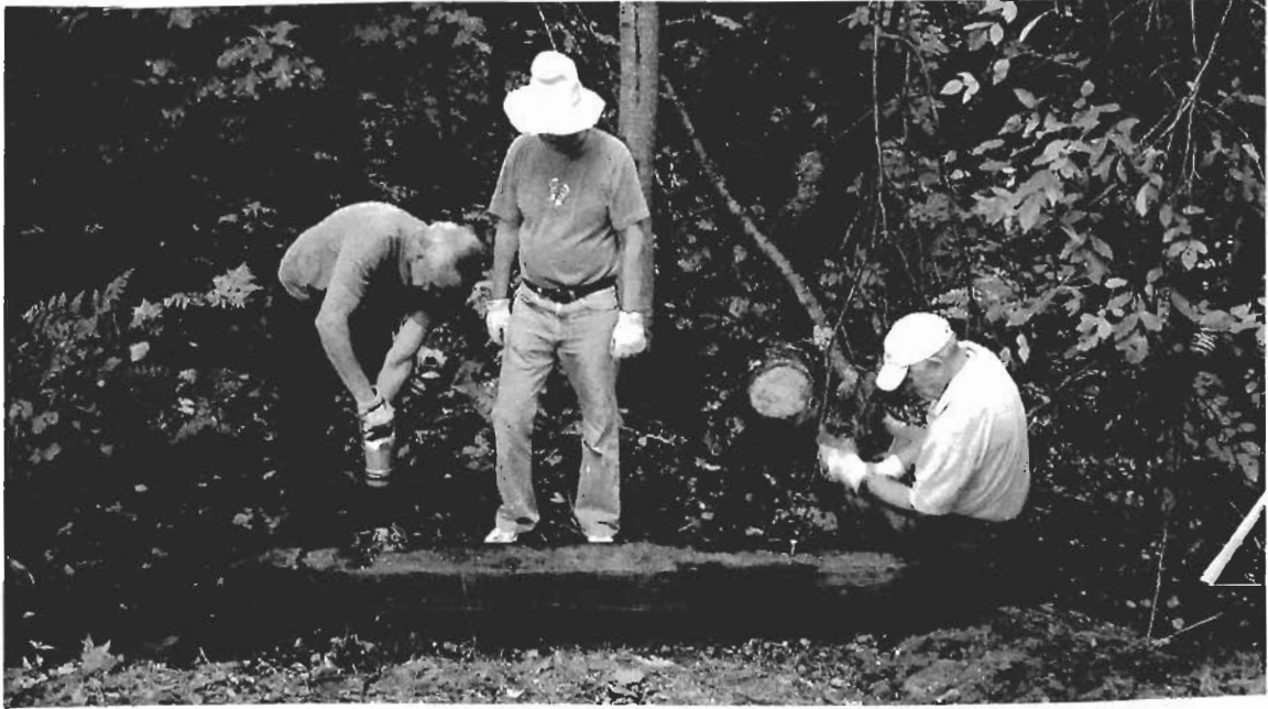
Constructing the railroad tie "bumpouts" for the benches was hard, hot, dirty work. Here Phil Mix (left) drills the holes, Moby Benedict pounds the spikes and Bob Condon supervises.
