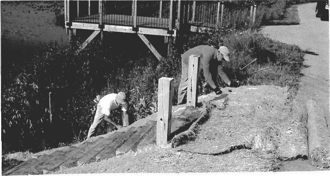
Pete Weir (left) and John Rothaar place the Ero-Mat around the new steps on the Elberta Causeway to prevent erosion
