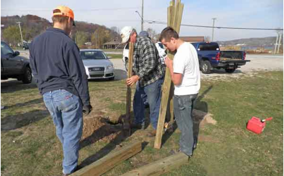
Mike Kaskinen, Pete Nugent and Chuck Anderson help William Richardson place the kiosk William is constructing, as an Eagle Scout project, in the Elberta Trailhead.
